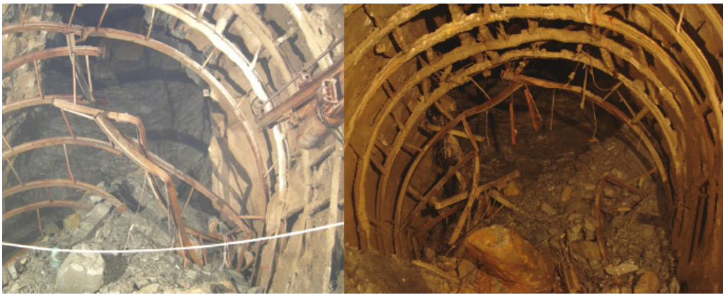
Figure 10: Huge collapse at crown because of mucking out the dropped material [28].
