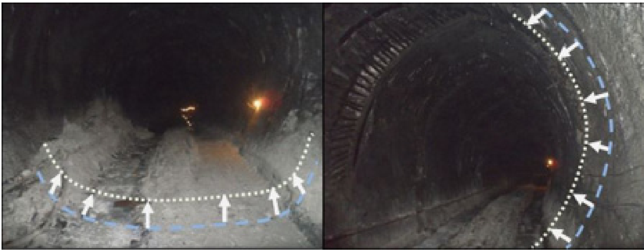
Figure 4. Tunnel squeezing in headrace tunnel of CHEP: Significant floor heave (left) and wall closure in hill side (right)
