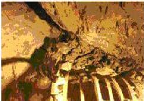
Figure 9: Front and Side view of over break Zone with exposed Steel sets of Ribs
