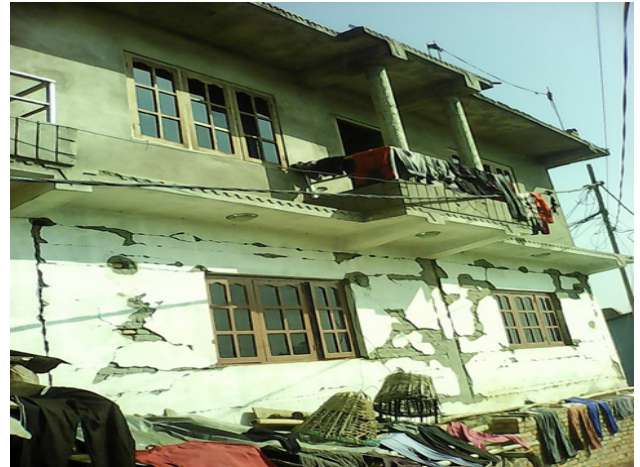
Figure 5: Structure Affected due to the Earthquake
