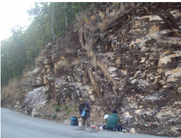
Fig. 3 Showing discontinuities along road cut section at location Fg1.
